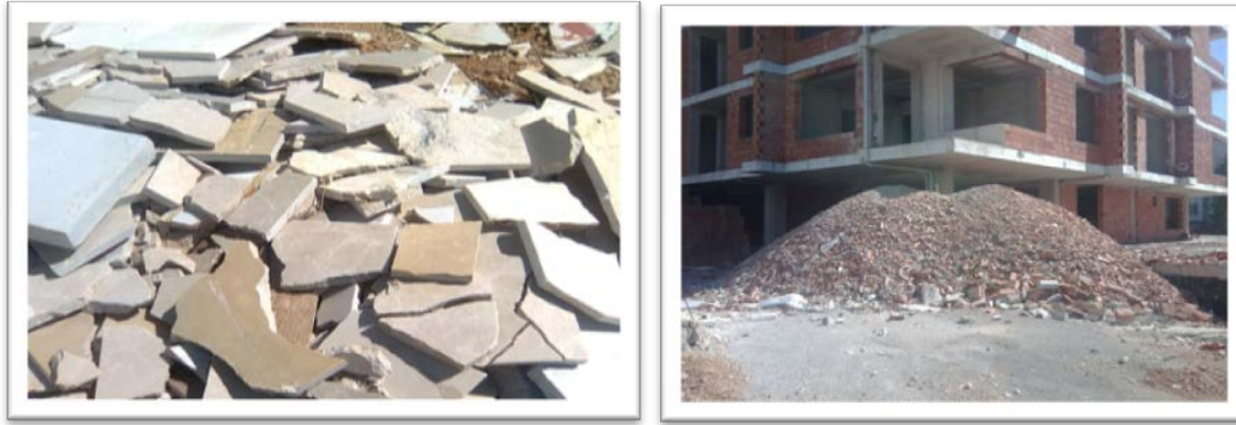
Figure 1: Wastes disposed in the construction site
